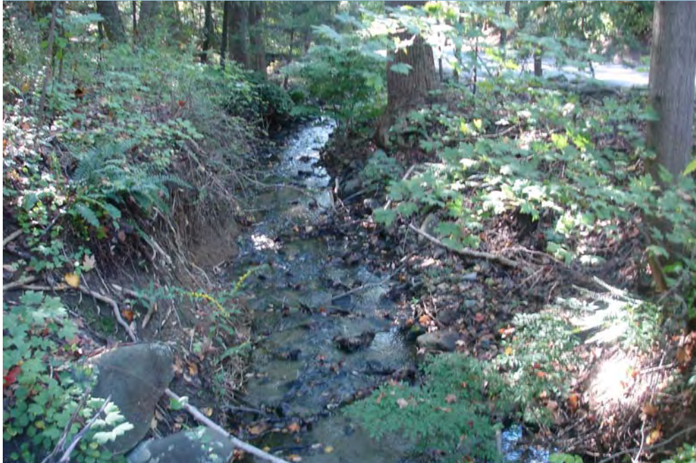
Figure 3-9. Eroded streambank on Quaker Bridge Road, Cortlandt
