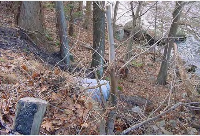
Figure 3-7. Untreated outfalls leading to Croton River.
